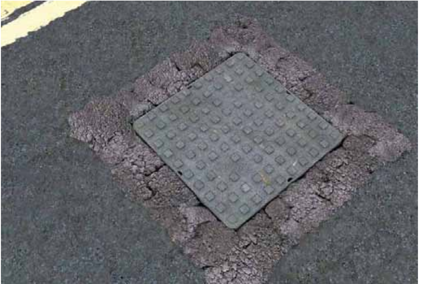
Stage 1 - Failed Manhole
